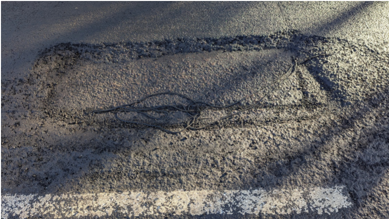
Cable exposed by pothole
