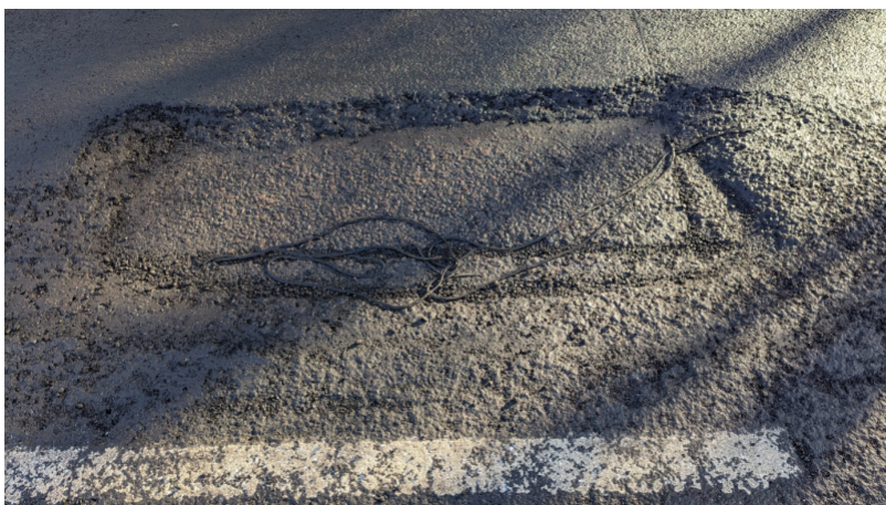
Cable exposed by pothole
