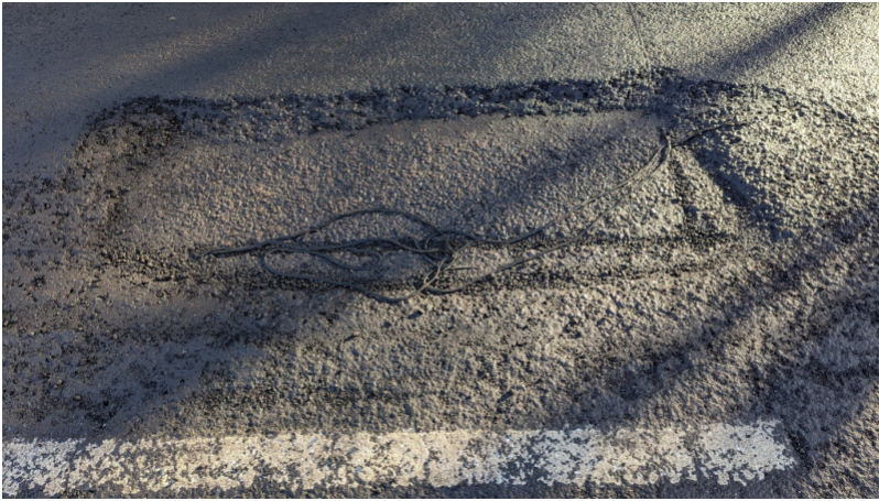
Cable exposed by pothole
