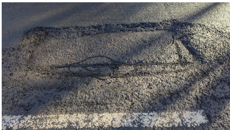
Cable exposed by pothole
