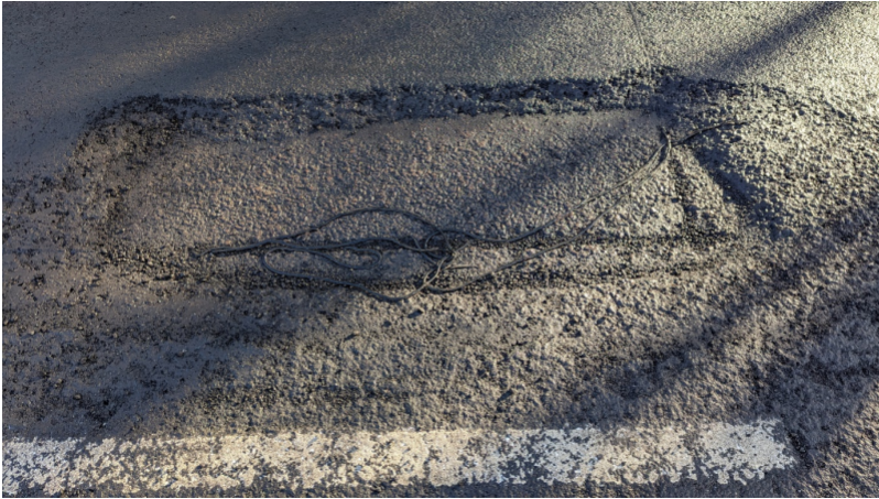
Cable exposed by pothole
